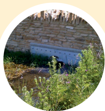
2. At Milton Street a flow control structure was built across Waterloo Brook. This protects Milton Street and cuts off the flow of water onto London street.
