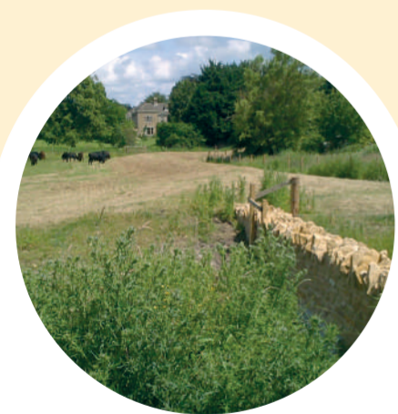
1. In Waterloo Meadow an earth bund was built. This protects Milton Street and cuts off the flow of water onto London street.
